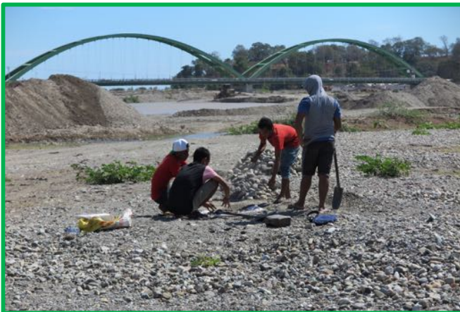
The new bridge over the Tono River – my staff doing their excavation work, by hand, for grit and pebbles.
