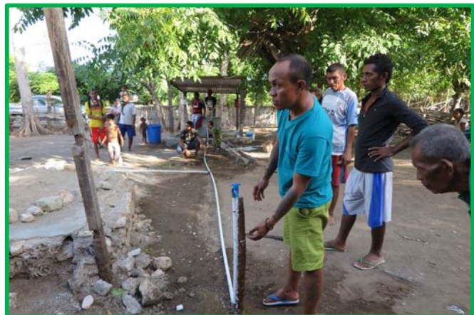
Water from a tap! The pipes have since been buried
